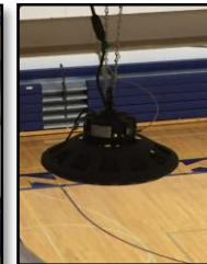
New LED fixture
